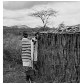
Maso Munyere, a young Maasai woman, builds her first house. Maso learnt the necessary skills from watching her mother. Photo: Practical Action / Lucky Lowe.
