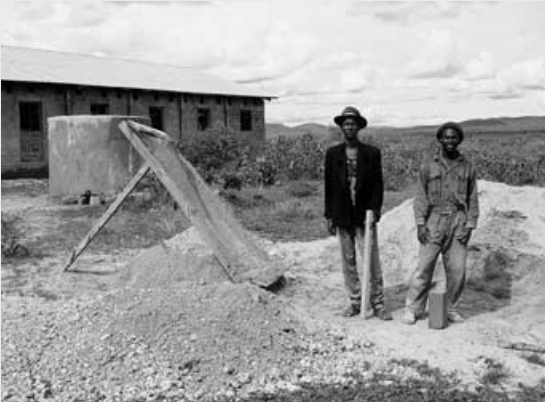
Amos Sikishoi and his assistant Olongida Molel in front of the new girls' dormitory being built at Ibisil Primary School. Photo: Practical Action.
