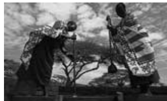
Maasai women being trained whilst preparing and moulding rammed earth walling. Photos: Practical Action / Neil Cooper.
